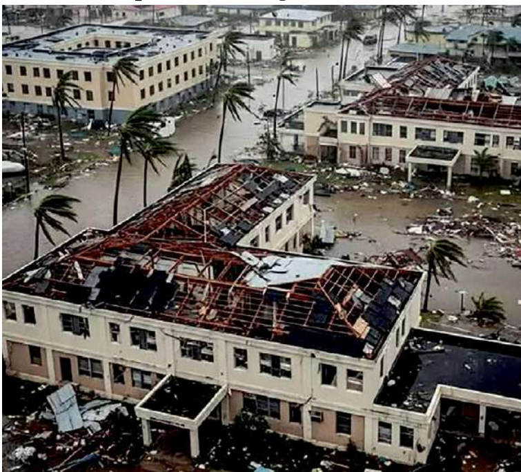
Damage to the Black River Hospital in St. Elizabeth was extensive. (Facebook image)
