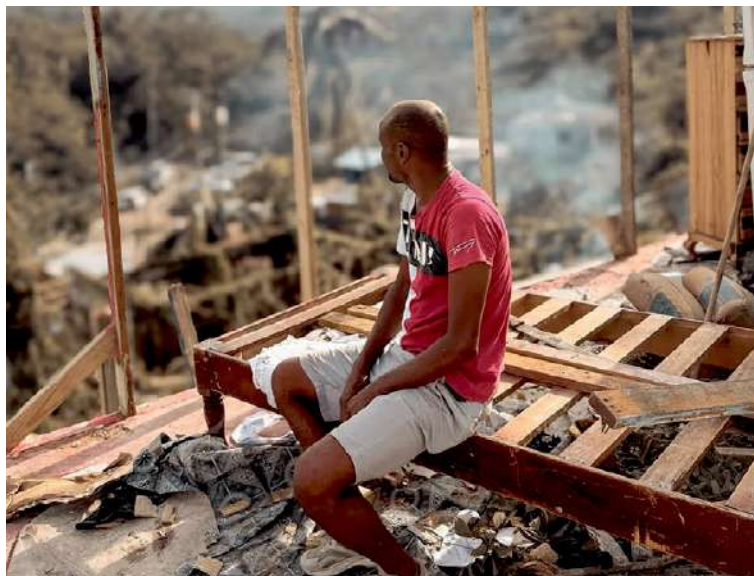
A resident of St. Ann, Jamaica, sits on a bare mattress frame, surrounded by the wreckage of his home after losing his roof and all his belongings in the storm. (Facebook image)
