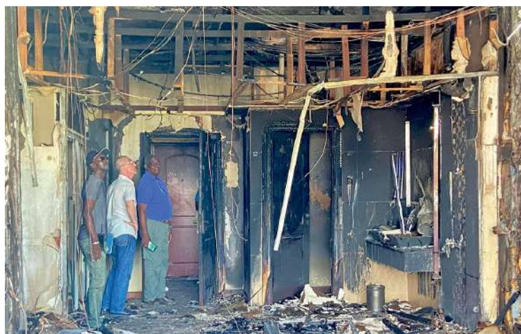
Fire officials inspect a hotel room at The Ramada Georgetown Princess Hotel, damaged by the fire on Sept. 23, 2023. (CMC image)
